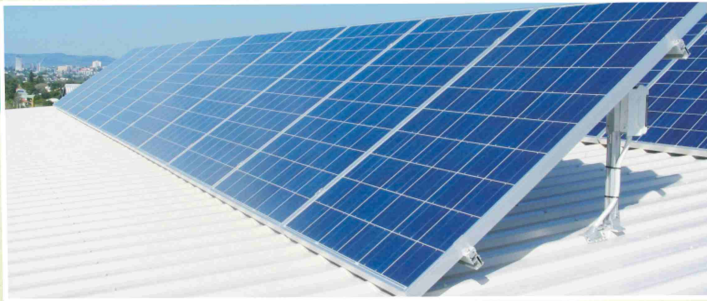
Solar Panel Installed
